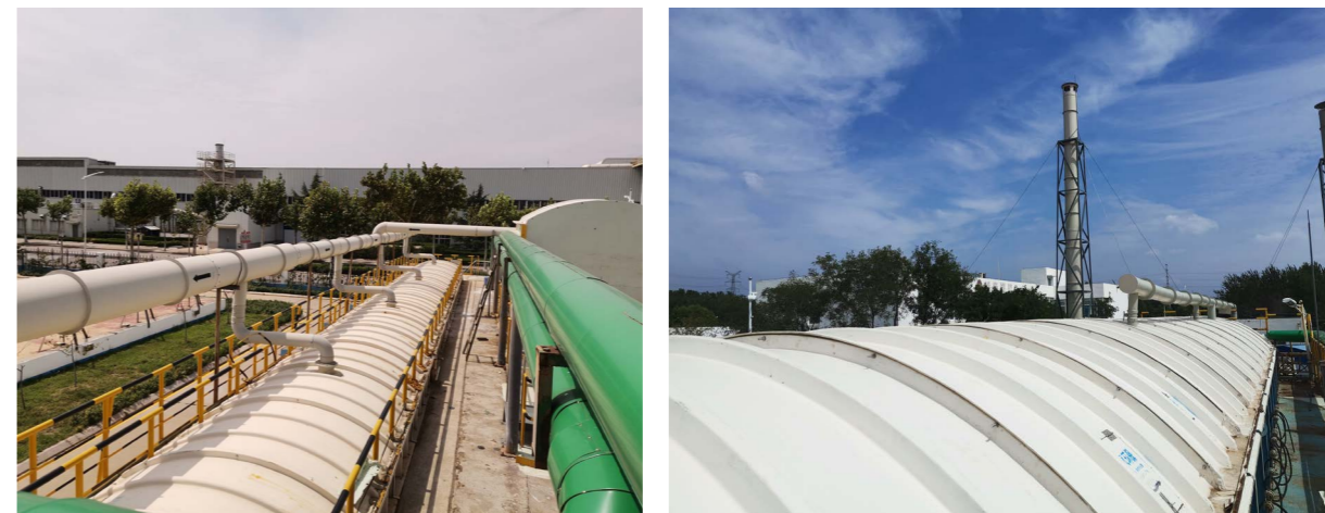
Collection and treatment of foul gas from the sewage station in the High-tech Park to ensure that no odorous gas escapes from the sewage station
