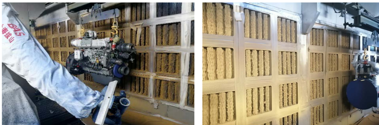
Renovating the dry spray booth to improve the adsorption and removal efficiency of spraying exhaust gas, reducing the concentration of exhaust gas emitted
