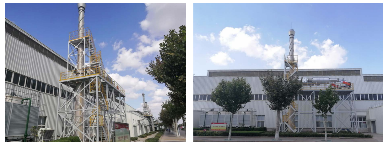
The facilities for treating waste gas emitted during trial run being put into use
