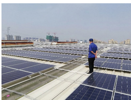
Photovoltaic power generation system
